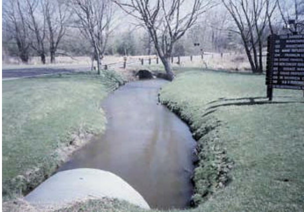
The status of existing infrastructure is an important factor in establishing a plan. To identify existing infrastructure, verify the location and type of culvert and upstream and downstream culvert size.
