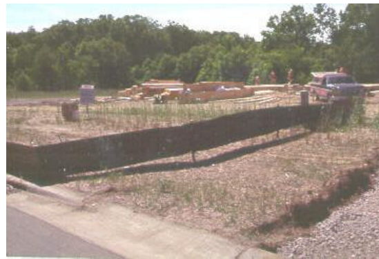
For sedimentation control, silt fences must be installed properly. The silt fence above is improperly installed because it is not trenched into the ground.
