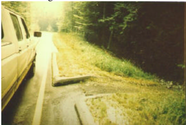
Direct stormwater runoff to stormwater retention and infiltration systems. Do not create direct channels from streets for stormwater to enter natural systems.
