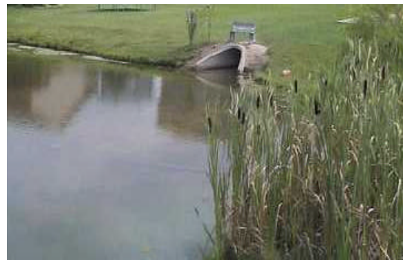
Detention basins are constructed systems that temporarily store water before discharging into the water body. The water discharges from the basin at a rate that will not increase flooding conditions in the stream.
