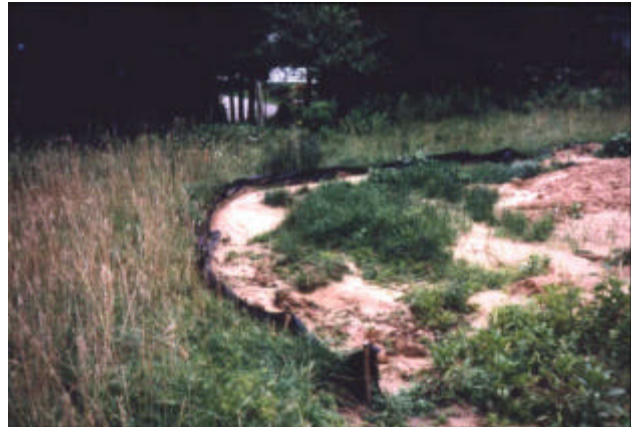
Utilizing a series of Best Management Practices is important to minimize runoff. In the picture above, a silt fence and buffer strip are used together to minimize the amount of sediment being swept off the site during a rain event.
