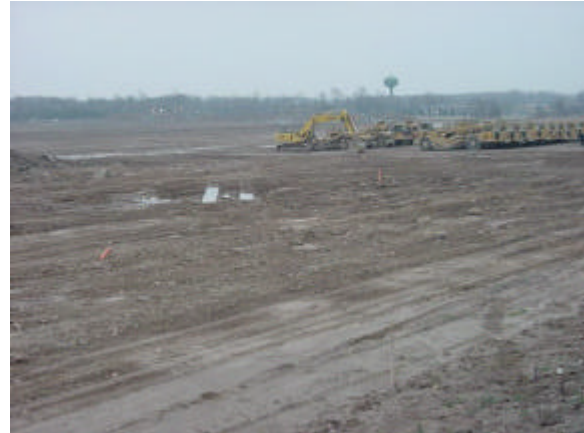
As a consequence of development and sprawl, many communities are experiencing degradation of their water resources. Stormwater runoff can carry contaminants that can pollute lakes and streams, and pose a threat to the health of people exposed to these degraded resources.
