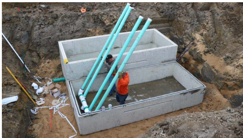
Figure 2. Inlet pipes being laid in the bottom of an iron slag filter. Drainage water enters at the bottom, moves up through the iron slag material (not yet installed) and leaves out a pipe near the top (not pictured) that leads to a nearby surface drain (not pictured). Photo credit: Macatawa Area Coordinating Council.
