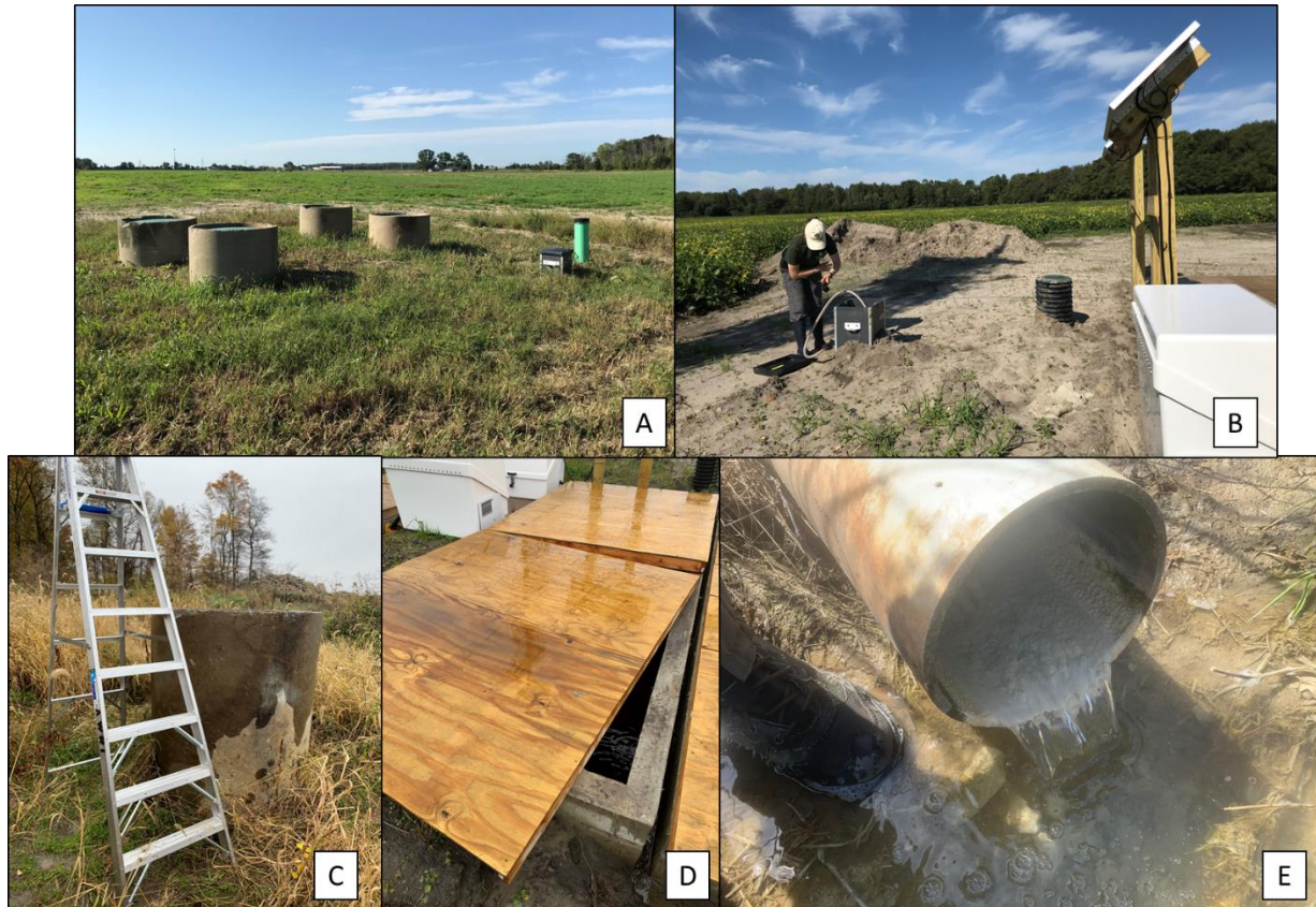
Figure 4. Photos of different sampling locations. A) Behind Mill 1 with completed iron slag filters in place. The green tube (far right) is an inflow sampling port that was installed only at this location. Access ports (for cement upright tubes) are for two slag filter basins (considered to be one slag filter site) that receive tile drain water from the adjoining field (in background) and are used to sample outflow. B) Sampling via a hand pump siphon to sample from a below-ground control box (inflow) at Fillmore Flex; Oak Grove 2 has a similar constructed inflow access (not shown). C) Slag filter outflow access point for Oak Grove 2, which required a ladder to remove the large plastic cap to sample outflow water. D) Slag filter outflow access point at Fillmore Flex, which is covered with large plywood lids. E) Outflow pipe at Behind Mill 1 directly after installation; the white particulate residue inside the tube is from the calcium carbonate layer placed on top of the iron slag inside the tanks to balance pH. Photo credit: Maggie Oudsema.
