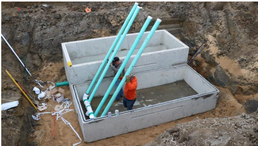
Figure 3. Inlet pipes being laid in the bottom of an iron slag filter. Drainage water enters at the bottom, moves up through the iron slag material (not yet installed) and leaves out a pipe near the top (not pictured) that leads to a nearby surface drain (not pictured). Photo credit: Macatawa Area Coordinating Council.
