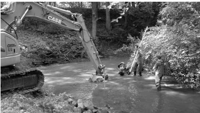
Heavy machinery was used to construct in-stream erosion controls in Sand Creek near Marne, Mich.
