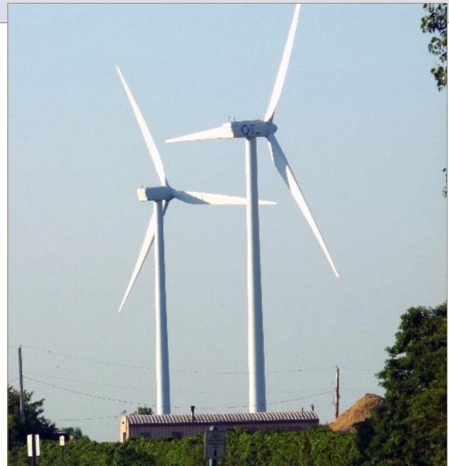
A pair of 1.8 MW wind turbines, Bowling Green, OH. (E. Nordman)
