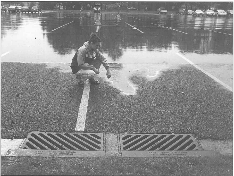
Parking Lot C strip of permeable asphalt after a rain. Note no storm water is reaching the outlet drains.
