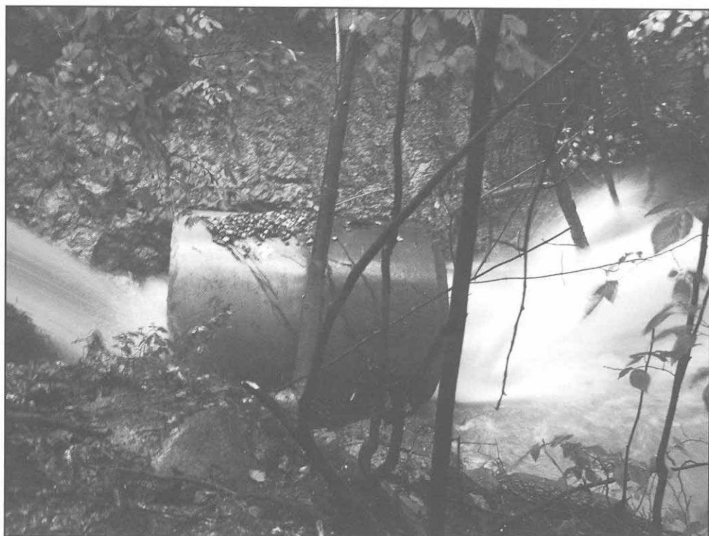
Discharge pipe near the Ravine Apartments taken during a rain event September 23, 2006.
