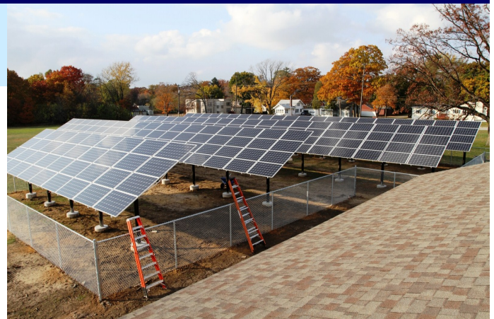
The new 70kW photovoltaic solar energy system recently installed at Every Woman's Place in Muskegon.
